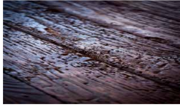
Figure 6. Damage by X. rufovillosum (URL6)
