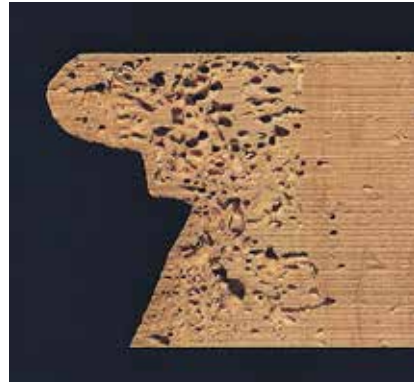
Figure 3. Damage by Anobium punctatum (URL3)
