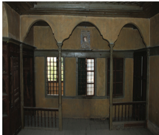
Figure 3. "Direklik" (decorated element between seki altı and seki üstü that includes timber posts, ornamented false arch and timber balustrade)
