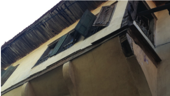
Figure 9. Physically deteriorated building elements
