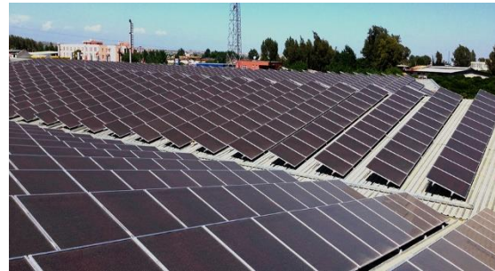
Fig.1 Orientation of PV plant, panels faces to south.
